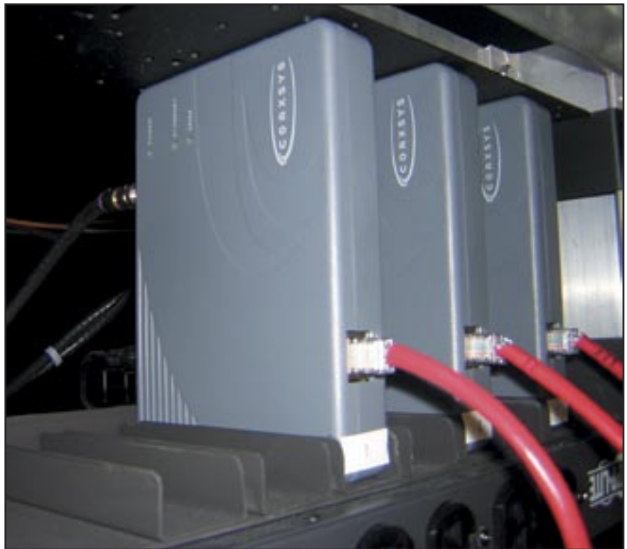
PurDigital's IPTV distribution closet: Three Coaxsys' TVnet adapters receive the CAT-5 Ethernet feed, and the data is then distributed over coax through the back of the adapters.
